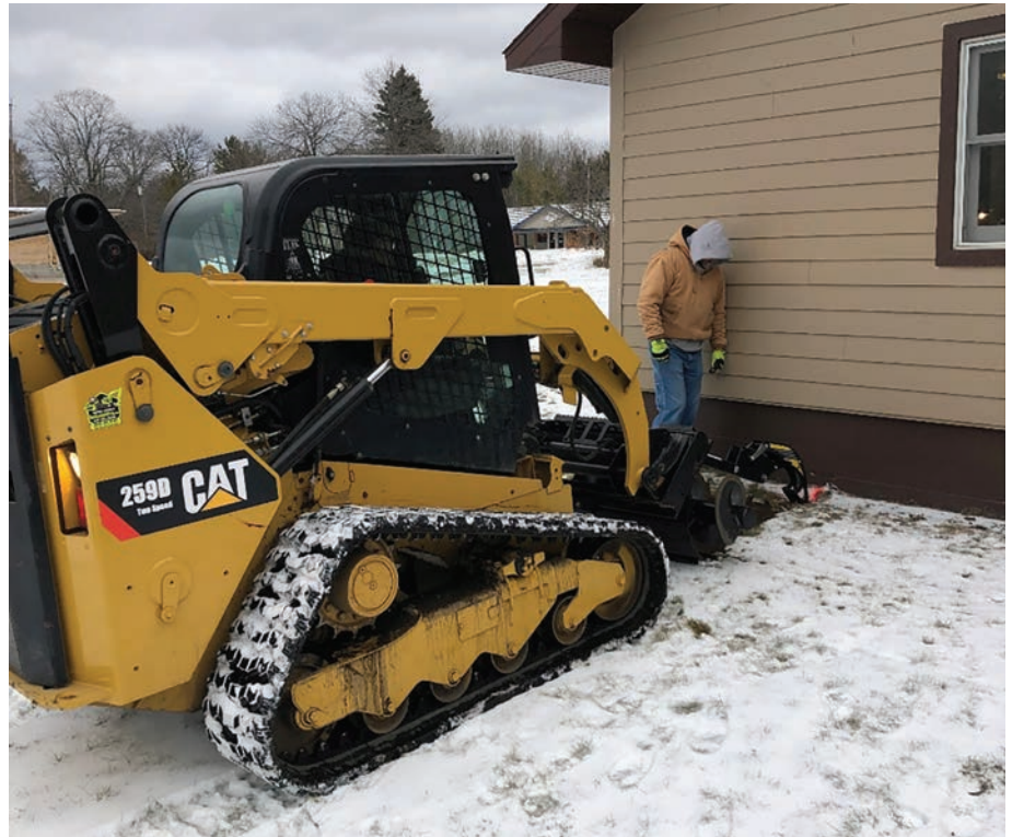
Pat Keehan guides Mike Jorgenson in the cooperative's new (used – grant procured) skid steer with trenching attachment for installation of conduit to get fiber feeds in and out of the cooperative. This machine will have multitudes of uses well beyond the fiber project. The common comment has been, "Why didn't we have one of these years ago!"
