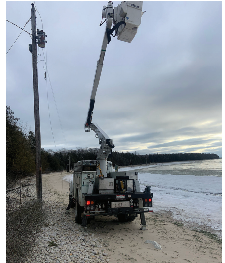
Believe me when I tell you that this is not our idea of a fun day at the beach, but we were lucky the ground was firm enough that we could get the truck to this pole to make repairs.
