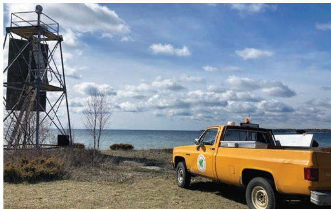
Marking live lines at the front range light.
