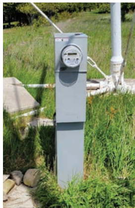
Meter pedestal installed in 2018 in anticipation of USCG cable failure as well as potential USF&W use.
