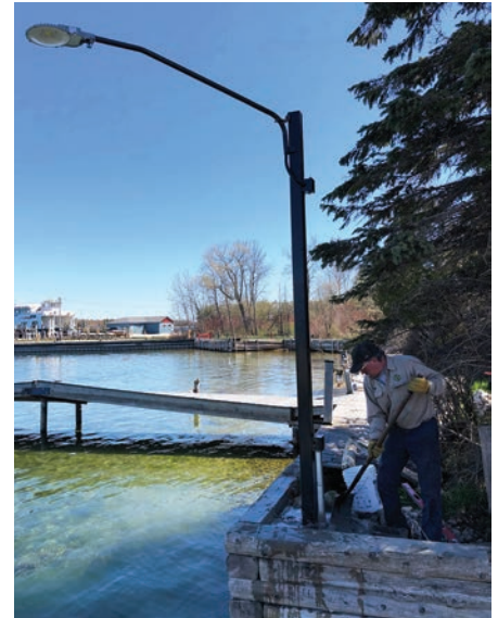
Mike Jorgenson levels cement at the base of the new launch ramp light built and installed by the cooperative.
