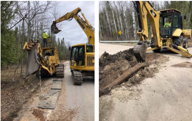
WIEC and Town of Washington crews worked together to install new culvert across Bay Point Road.
