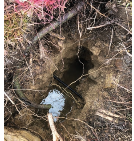
Underground phone line exposed by hydrovac excavator.
