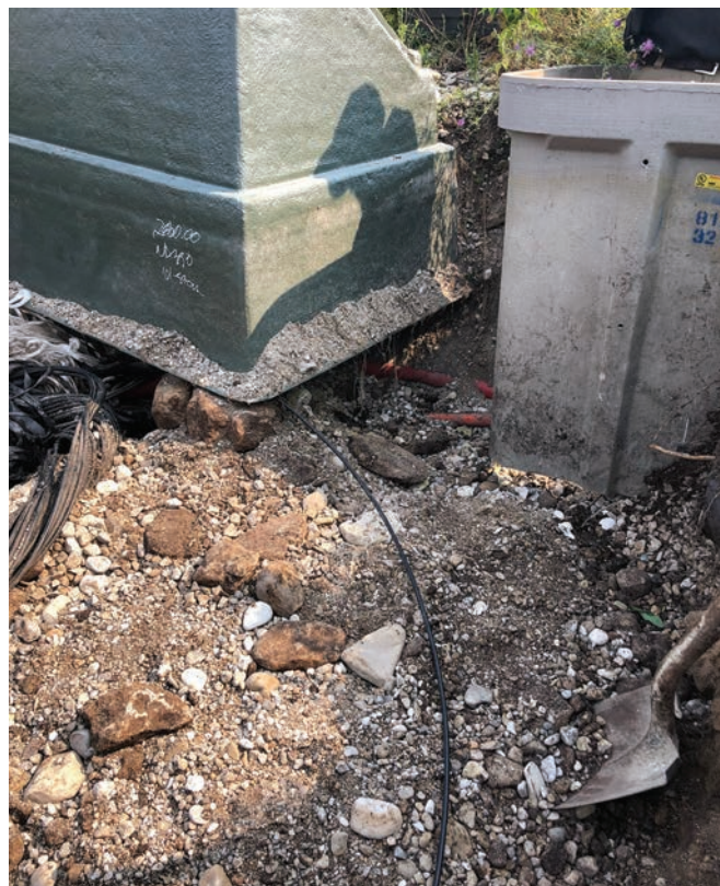
Excavated cabinets and exposed 24-strand fiber awaiting splicing. These cabinets were covered again, leaving a small trench to work in. This photo was taken before that happened.
