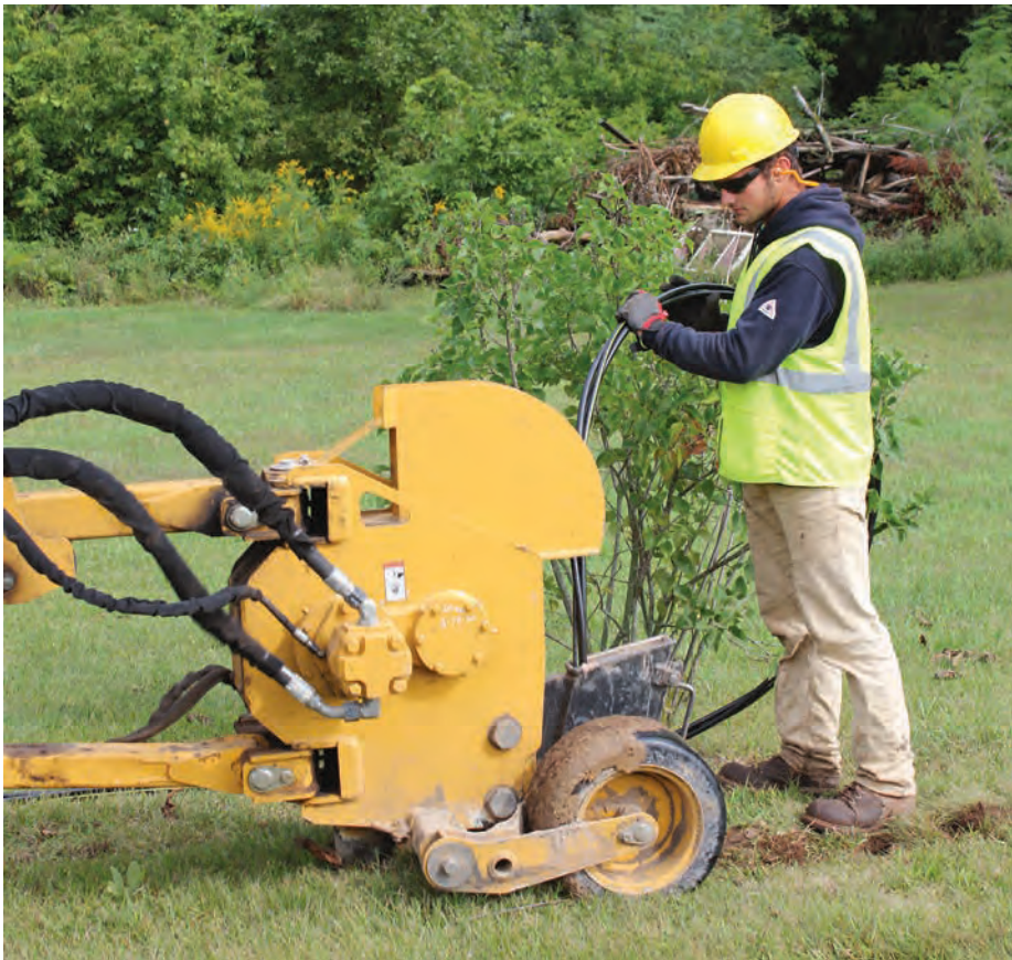
Oconto Electric Cooperative Apprentice Lineman Jake Baldwin demonstrates plowing in the underground cable. At this location, the cooperative was transitioning from overhead to underground powerlines. Photo courtesy Katie Jagiello, Oconto Electric Cooperative
