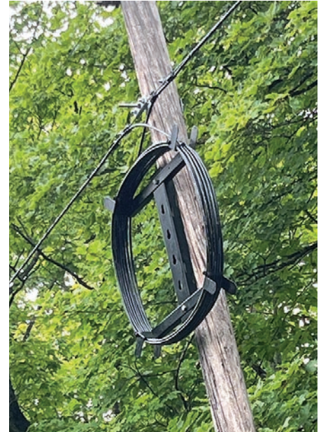
"H-frame" installation cleans up slack spans and splice locations of the fiber project.
