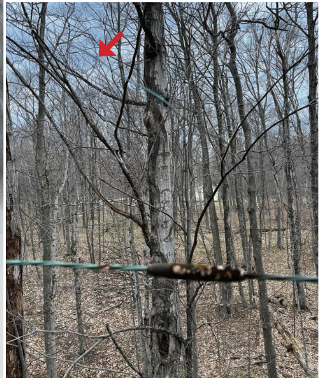
Damage from the April 2 storm continues to show up and require costly repairs. In this case, a stranded conductor (indicated by red arrow) was tapping into an existing splice, burning the splice and causing intermittent blinks.
