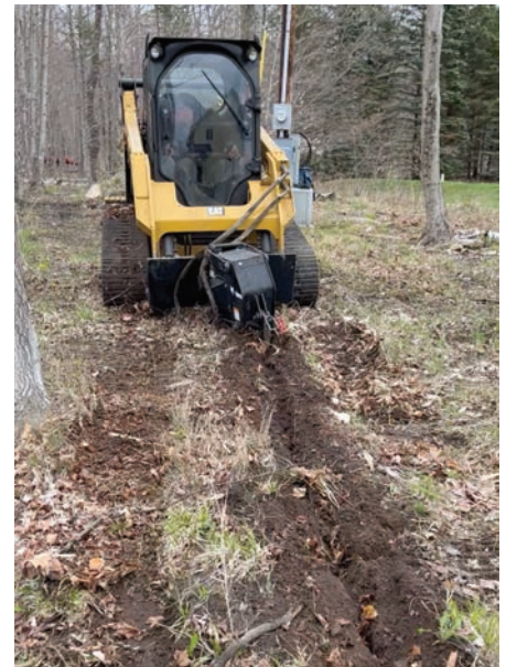
Mike kept up with plowing underground while Karcz was on other worksites.
